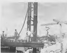
SIGNALLING the crane operator is Foreman Don McLean. The pile-driving ram travels up and down the attachment shows behind the pile.
